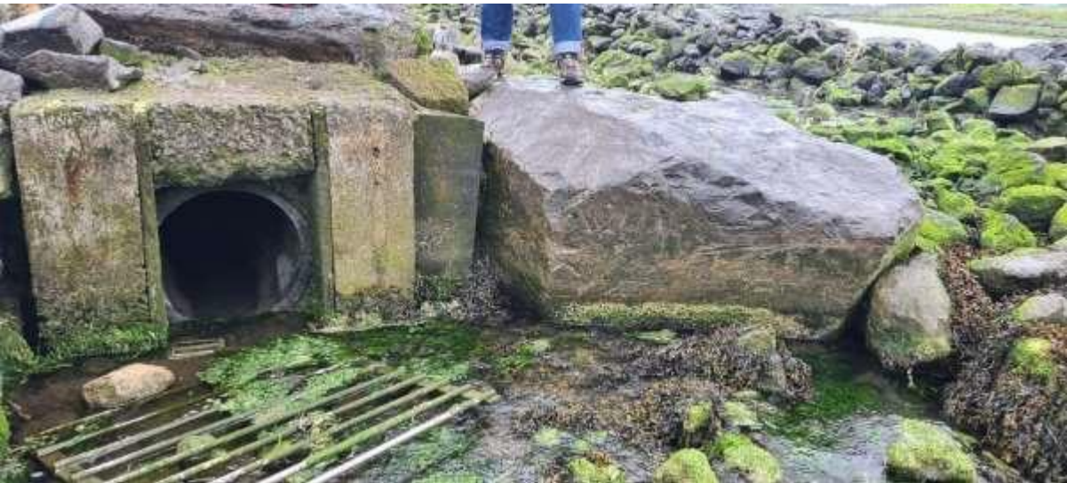
Oranmore Pump House Overflow pipe – May 2021
