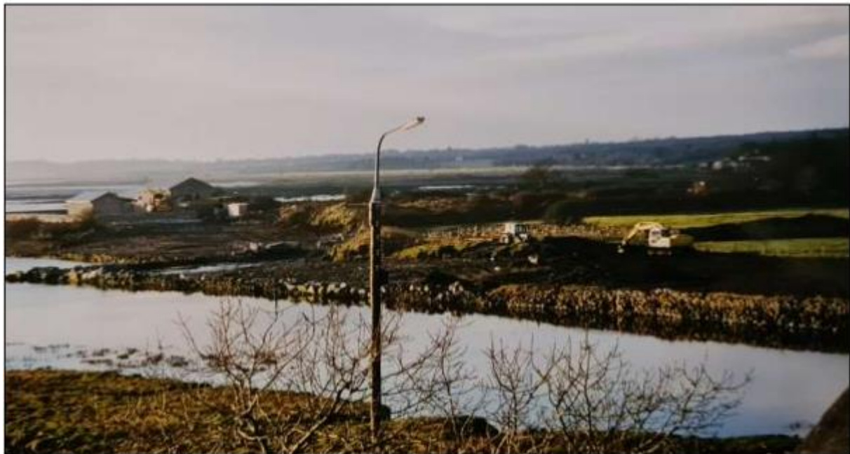
Open soil which was washed out numerous times by high tides during construction works
