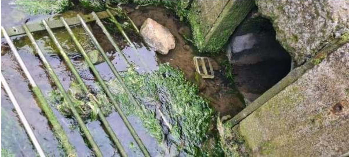
Oranmore Pump House Overflow pipe – May 2021
